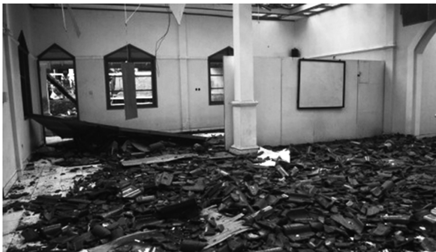
The condition of Nurhidayah Mosque belong to Ahmadiyah followers after destruction in Cisaar, Cipeuyeu, Cianjur, West Java, on Saturday, February 8th, 2012. (Picture: TEMPO/Prima Mulla).
