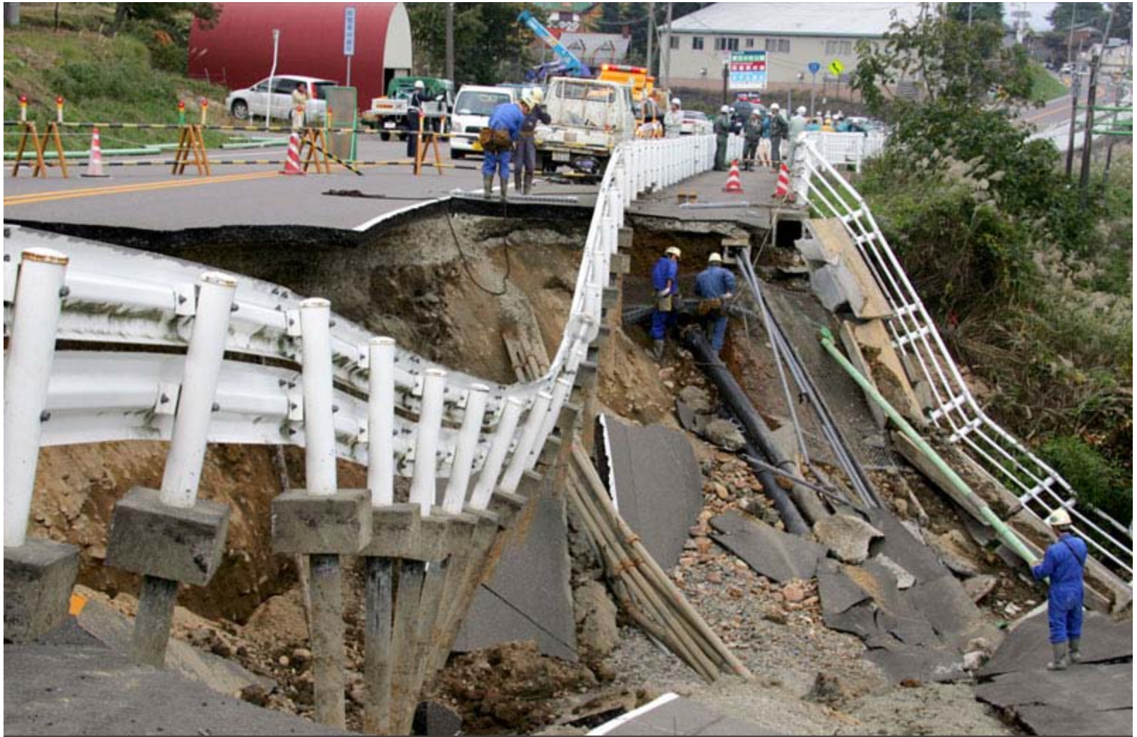
Aftermath of an earthquake in Japan, 2004 Photograph by Kimimasa Mayama/Reuters
